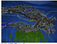
Cable C09, Photo - 5
